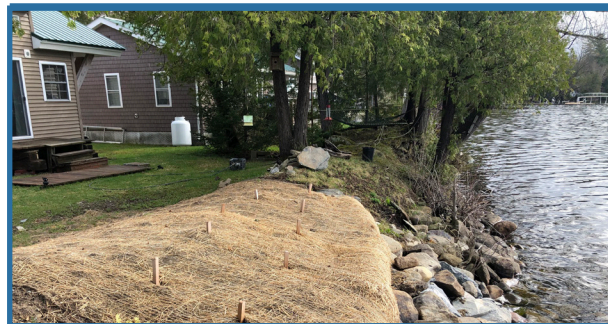
Above: A Lake Carmi shore restoration project funded through the Missiquoi Bay Clean Water Service Provider. Concrete blocks on a lakeshore property were removed and replaced with native vegetation.
