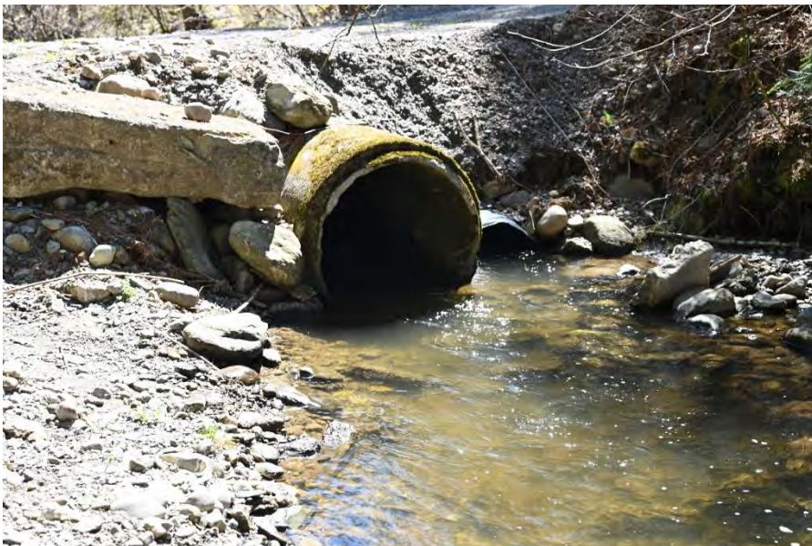
Figure 68. View southeast of the outlet side of the culvert that carries Trout Brook under the west access road.
