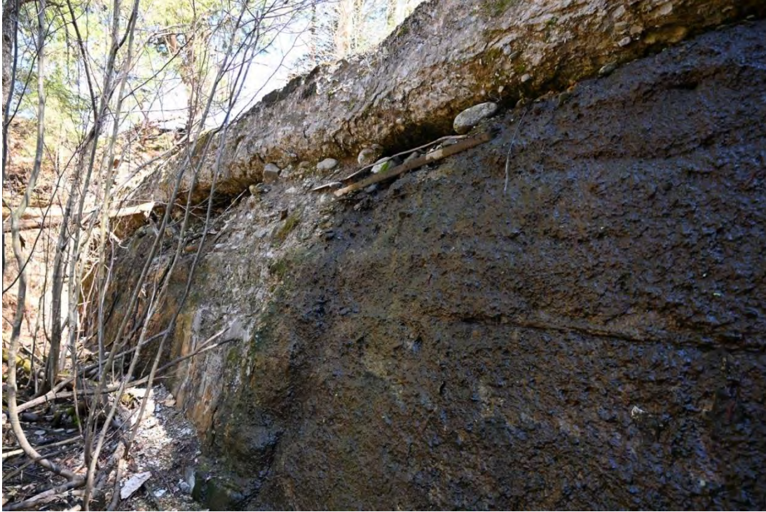
Figure 45. View of the left side of the main dam's downstream face, looking west.
