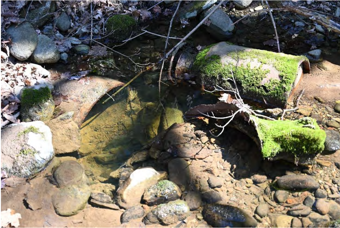
Figure 53. View of iron pipe / possible “blow-off pipe” south of the gate house and control chamber on the left side of the spillway.
