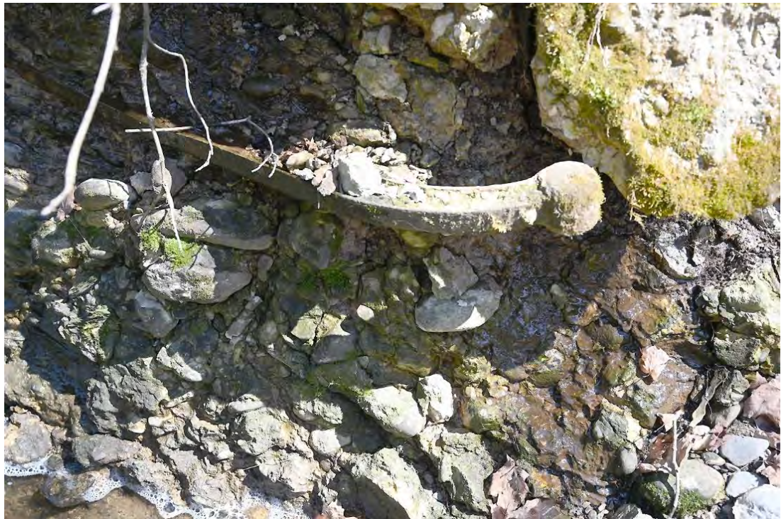
Figure 55. View of an exposed metal reinforcement element embedded in the right apron wall.
