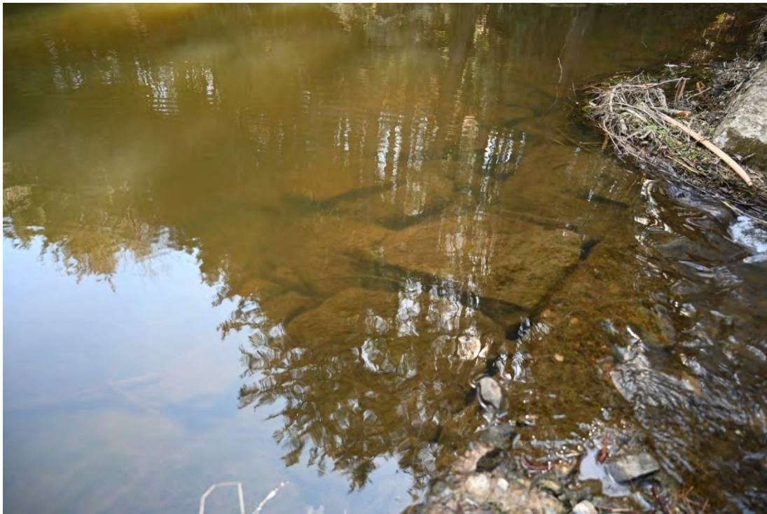
Figure 57. View of the pavement feature on the upstream side of the dam, looking northeast.
