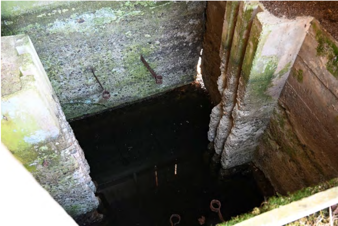
Figure 50. View of the interior of the gate chamber; note the concrete formed guides for the copper screens and the metal gate thread guides.
