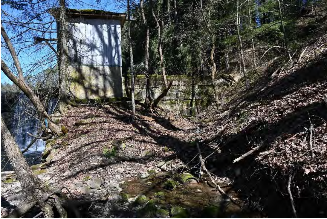
Figure 51. View of the gate house and control chamber on the left side of the spillway, looking west, note bracket on back of structure.
