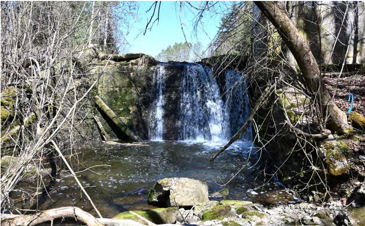
Figure 38. View of the spillway and apron area of the main dam, looking north.
