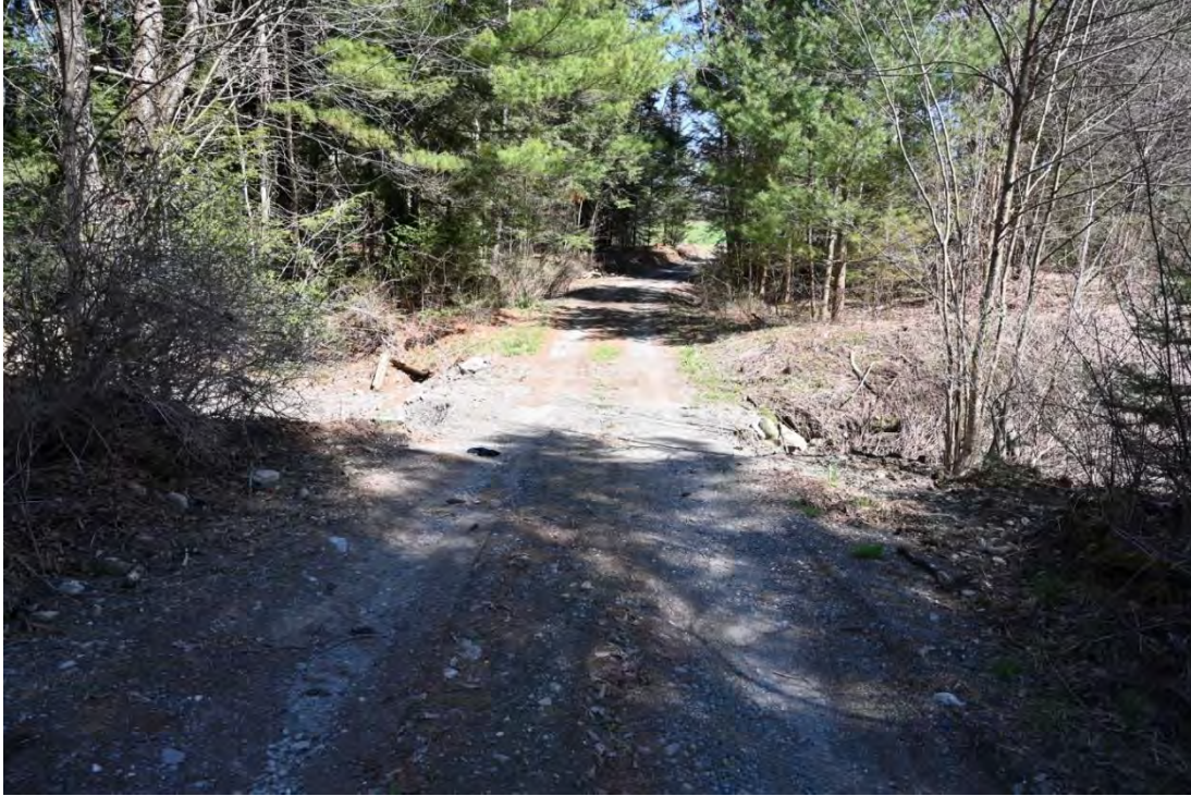
Figure 15. View of the culvert crossing Trout Brook on the proposed western access route, looking north.
