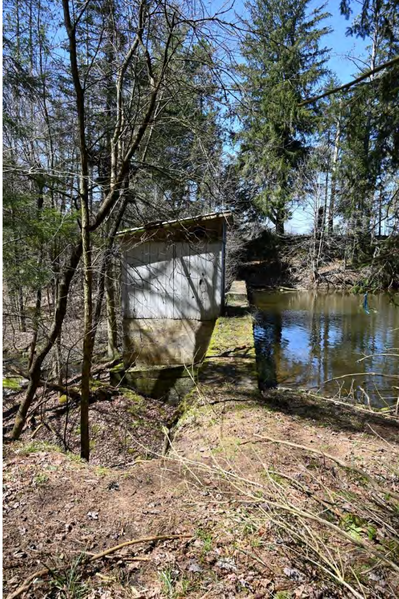
Figure 48. View of the gate house and control chamber on the left side of the spillway, looking west.
