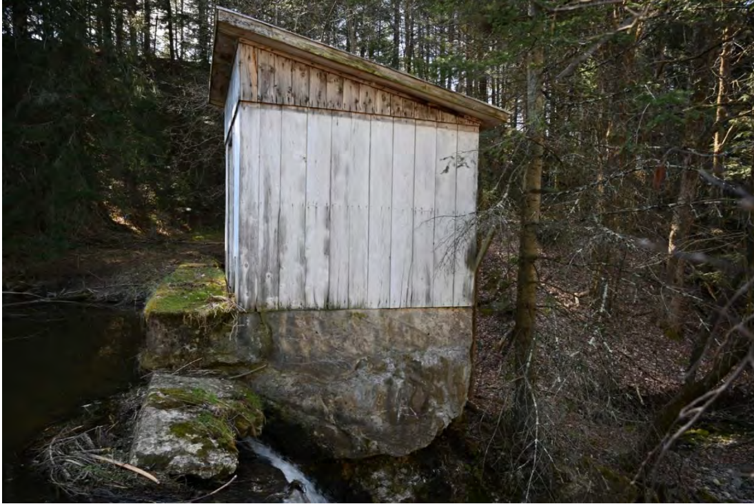
Figure 46. View of the gate house and control chamber on the left side of the spillway, looking east.
