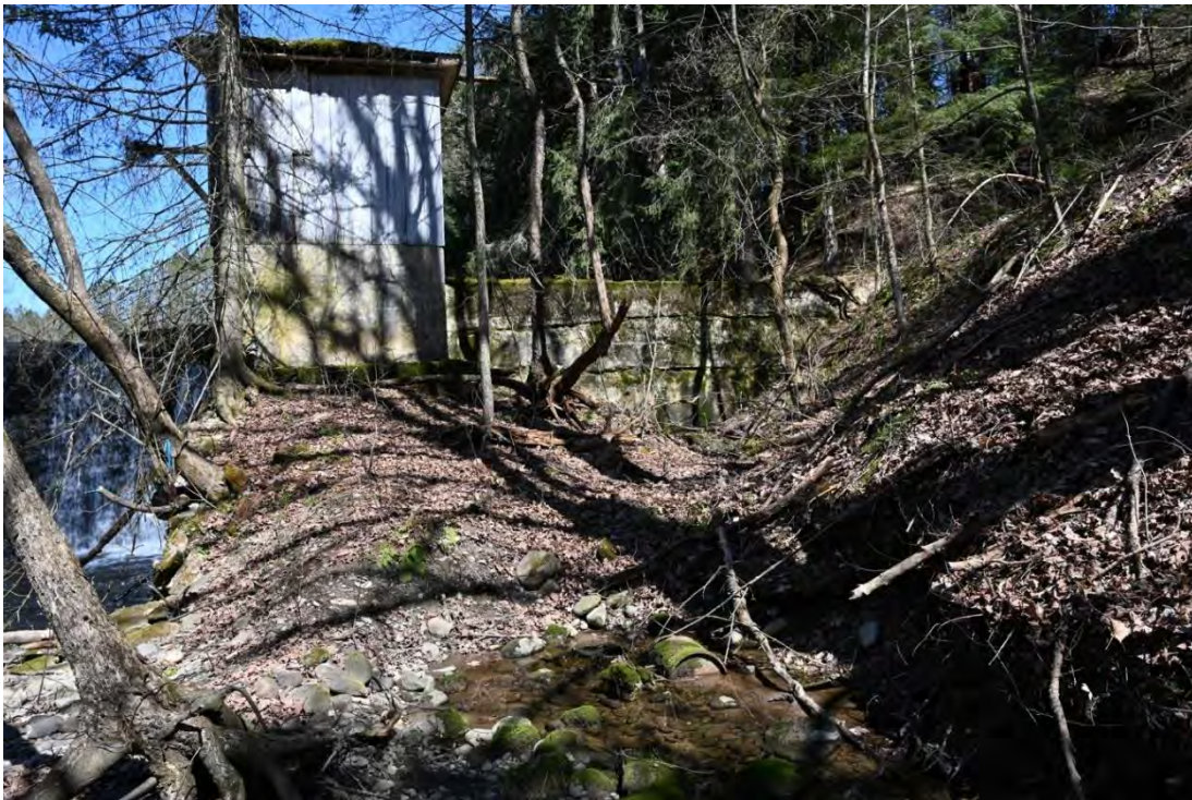
Figure 47. View of the gate house and control chamber on the left side of the spillway, looking north.
