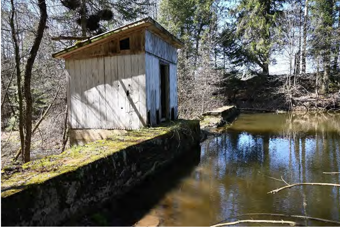
Figure 49. View of the gate house and control chamber on the left side of the spillway, looking west.
