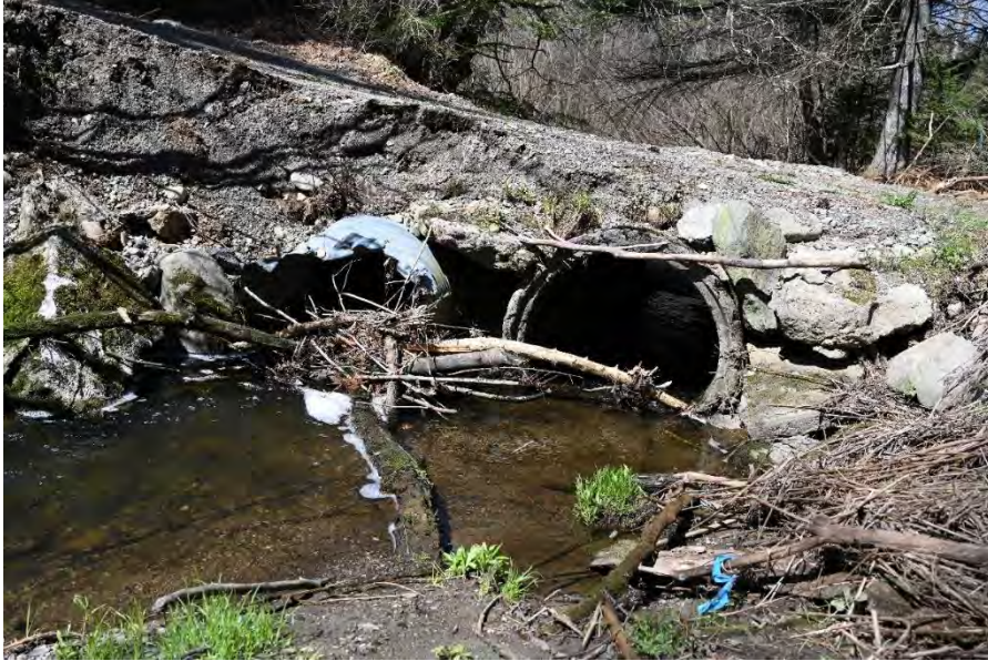
Figure 67. View southwest of the inlet side of the culvert that carries Trout Brook under the west access road.
