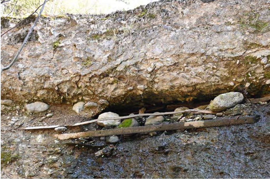
Figure 54. View of exposed metal reinforcement elements on the left side downstream face of structure; also note the concrete aggregate sizes and volume.
