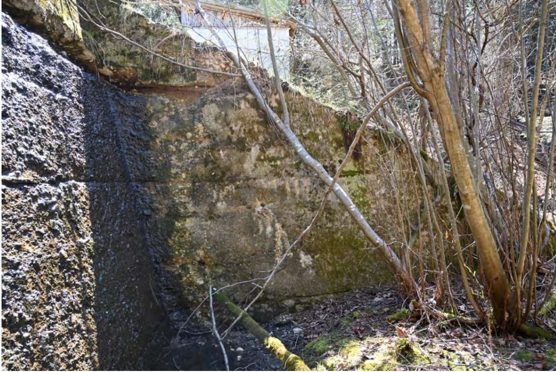
Figure 43. View of the outside surface of the right apron wall, looking east.
