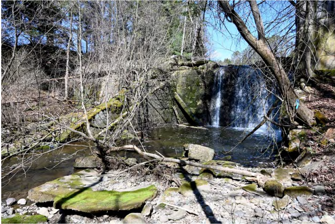
Figure 2. View of the downstream face of the Trout Brook Dam, looking north.
