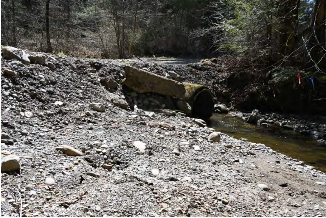
Figure 17. View of a cement culvert on Trout Brook and an extensive area of fill around it on the proposed western access route, looking southeast.
