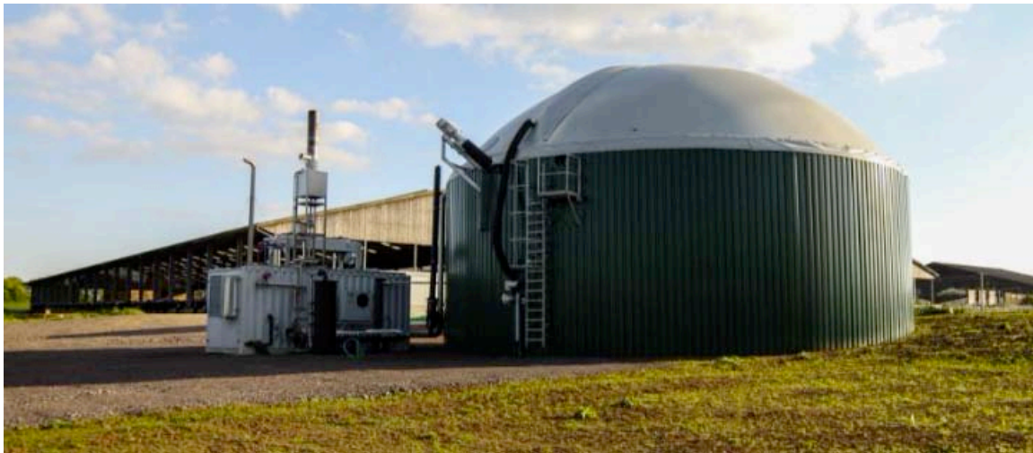
Photo of a similar project at a different farm showing the digester tank, generator with a flare mounted on the generator's roof.
