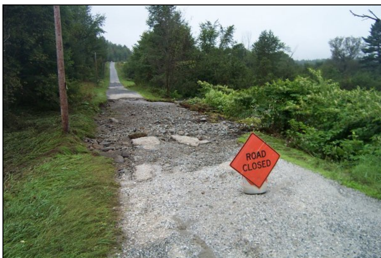
Photo courtesy of Henry Raymond August 29, 2004~Flooding closes the Fanton Road.
