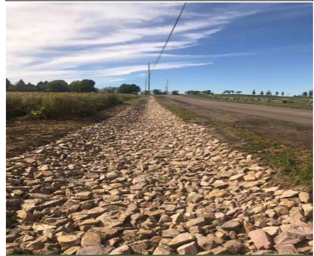
This new stone lined ditch on Kibbe Point Road was funded by Grants In Aid in 2022 and will reduce erosion and improve stormwater infiltration.
