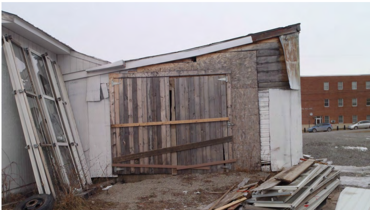
Photo 23: 14 Stebbins Street: Southern entrance to the warehouse building. Photo taken facing east by Sanborn Head on January 10, 2017.
