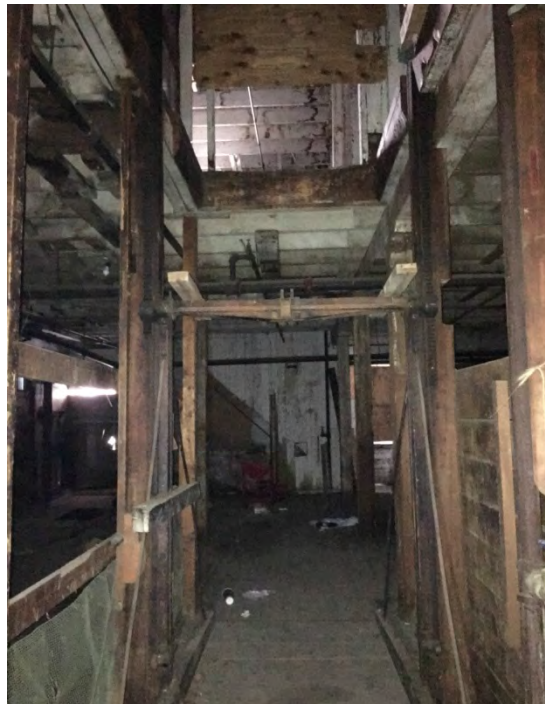
Photo 10: 14 Stebbins Street: A former lift was observed in the western portion of the warehouse building. Photo taken facing south by Sanborn Head on January 10, 2017.
