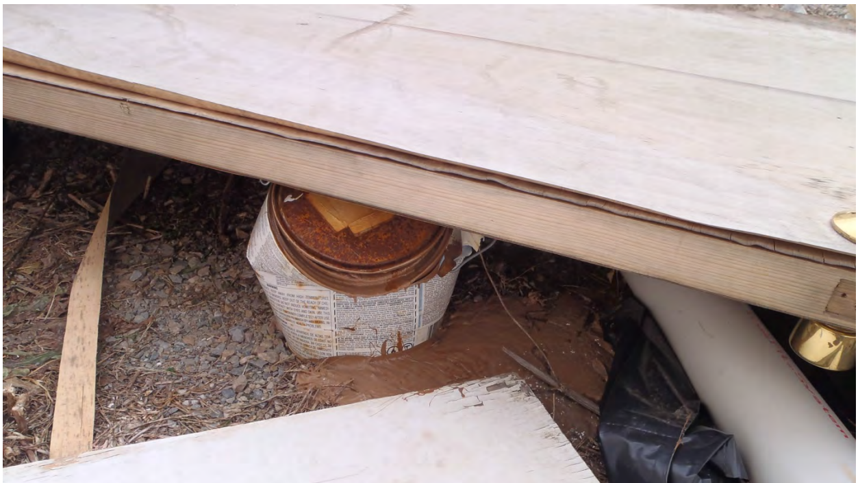
Photo 18: 14 Stebbins Street: A can of paint has spilled to the ground surface on the southern side of the warehouse building. Photo taken by Sanborn Head on January 10, 2017.
