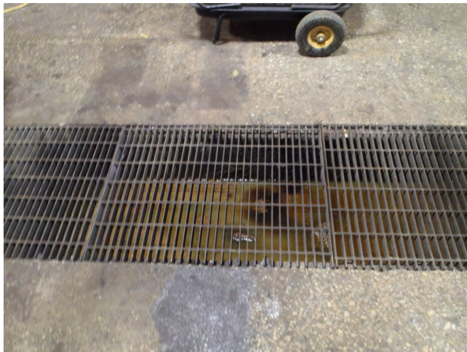
Photo 36: 21 Stebbins Street: A floor drain in the former car wash building; drain reportedly discharges to a 1,000-gallon underground grit trap in parking lot. Photo taken facing south by Sanborn Head on January 10, 2017.
