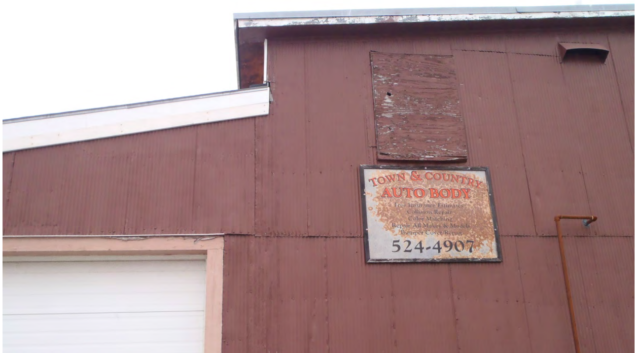
Photo 30: 23 Stebbins Street: The former Town & Country Auto Body shop is located at 23 Stebbins Street. Photo taken facing north by Sanborn Head on January 10, 2017.
